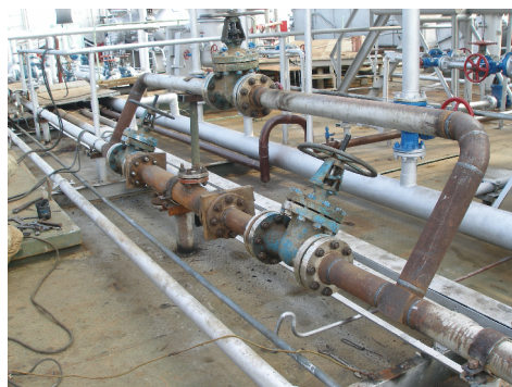
Figure 8. Photo of the pipe layout of field test facility manifold
